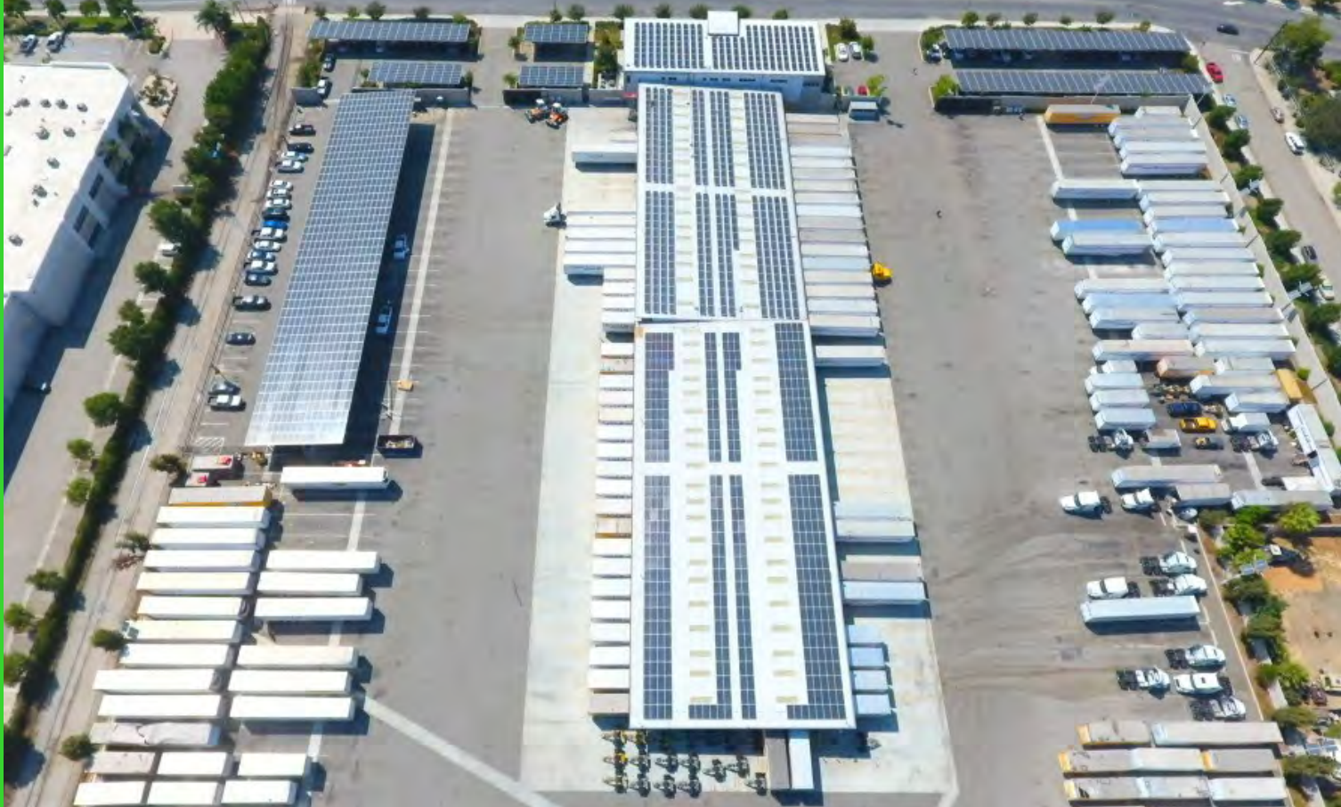
Caption: Dependable Highway Express installed solar panels and onsite energy storage at its shipping and receiving facility in Ontario, California.
